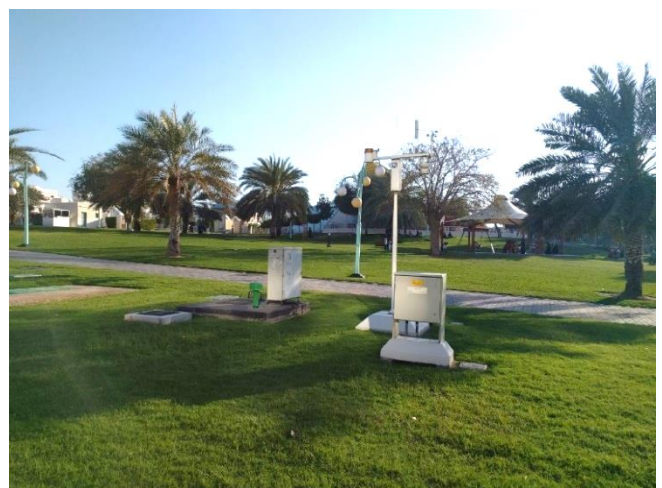
Tonick RM-2 and weather station installed in Abu Dhabi park.
